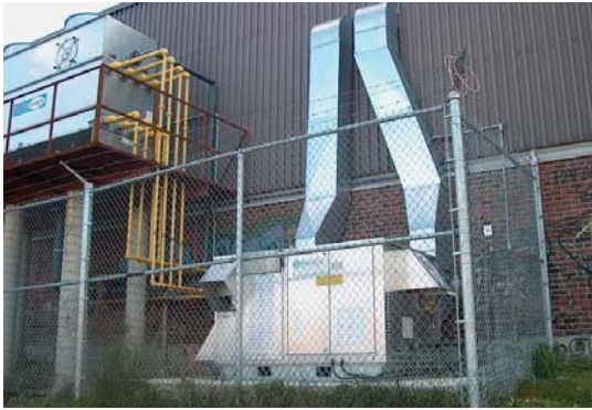
Desiccant dehumidification system at Campeau Arena in Gatineau
